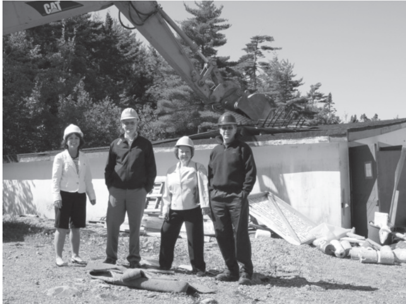
Debbie Hum, Sean O'Connor, Mary Wile and Mel Hackett are shown at demolition of Maskwa shed and start of construction of new Maskwa Canoe Club.
